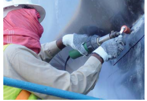
Welding a patch with TRIAC PID on a building site in Dubai.
